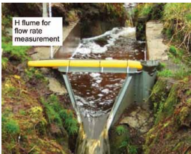
Figure 3: Monitoring station – H flume (maximum flow rate: 158 l/s).
