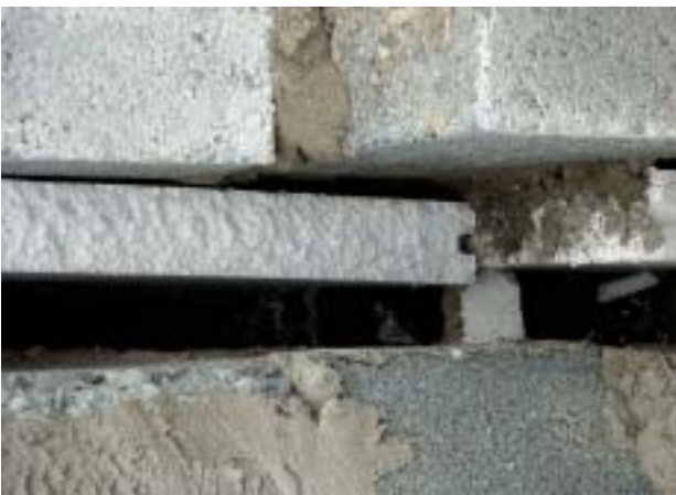
Figure 2: Mortar keeping insulation from the blockwork leading to significant air gap and thermal looping.
