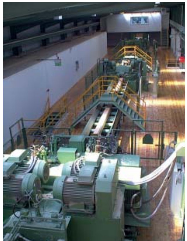
Figure 4: The new investment at Glennon (Bros.) Timber Ltd's mill in Fermoy, Co Cork epitomises the commitment of the Irish sawmilling industry to continued capital investment in state-of-the-art technology.
